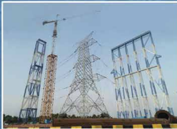
765 kV D/C TOWER
