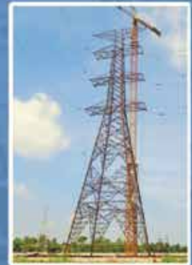
500 kv D/C TOWER
