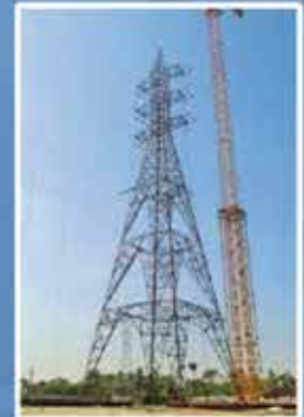
220 kv D/C Tower
