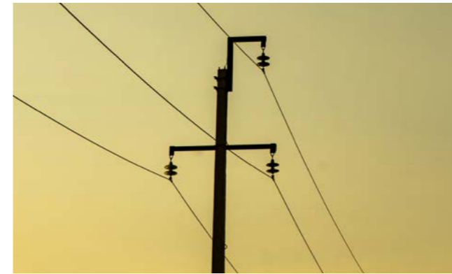
Power distribution poles
