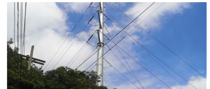
500 kV D/C - Tower
