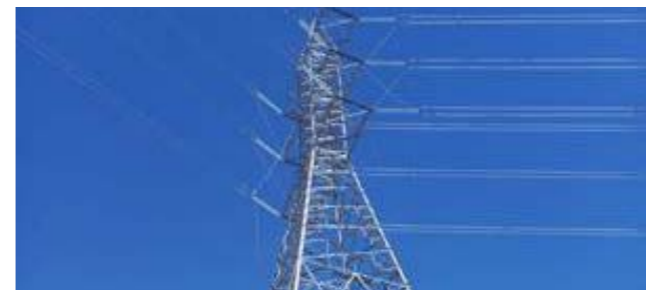
220 kV - D/C Tower
