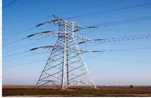
Power Transmission Tower
