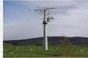
Power Distribution Poles
