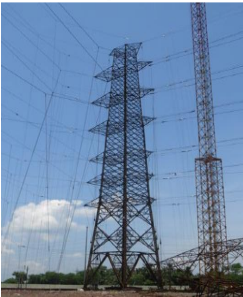
220kV Transmission Tower
