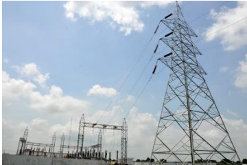
Transmission Line EPC
