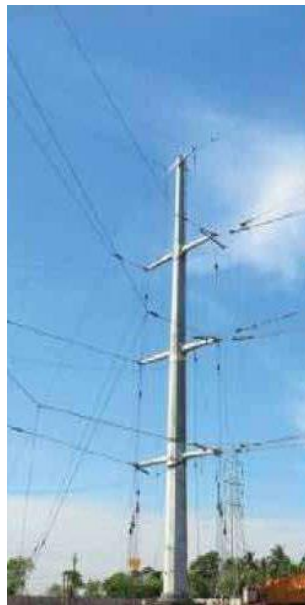
400kV D/C Quad Moose Monopole
