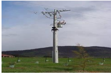
Power Distribution Poles
