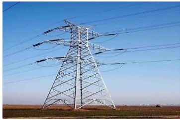
Power Transmission Tower
