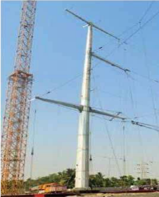
765kV S/C Monopole
