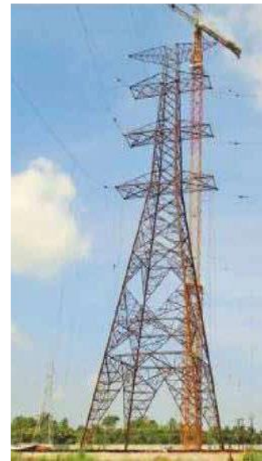
500kV Transmission Tower
