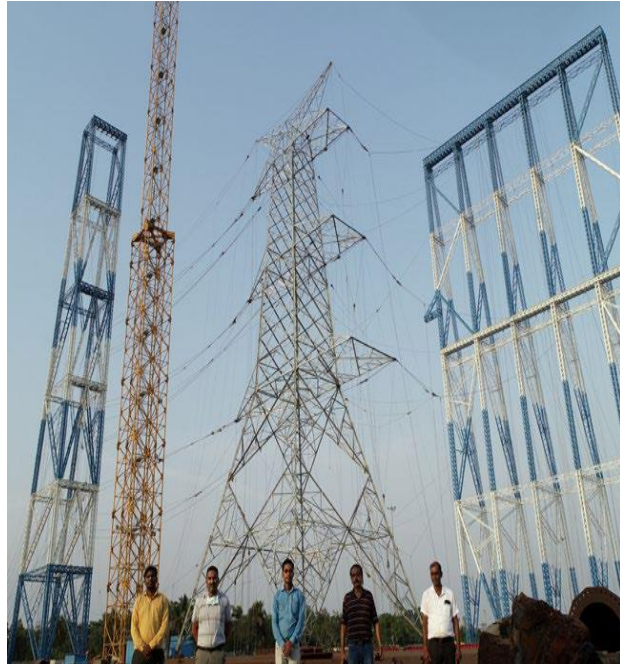
765kV Transmission Tower
