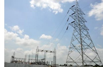
Transmission Line EPC
